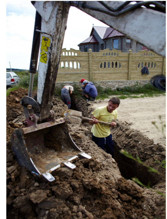
Photo courtesy of Skat Consulting Ltd.: Construction of a water supply system in rural Moldova. All households are individually connected.
